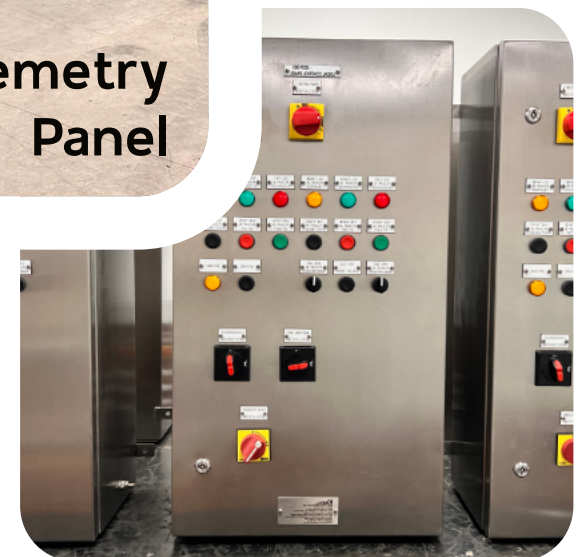
Local Control Panel
