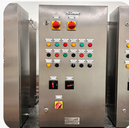
Local Control Panel
